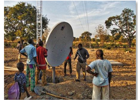
Figure 6: AMN base station in Benin. Source: VLN
